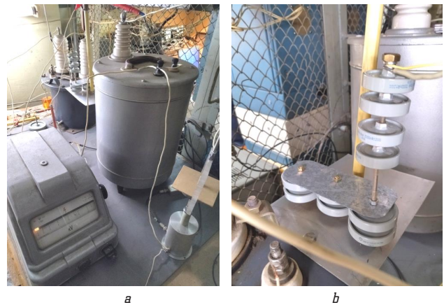
Fig. 2. General view of partial discharge: a – measuring installation; b – capacitor bank
