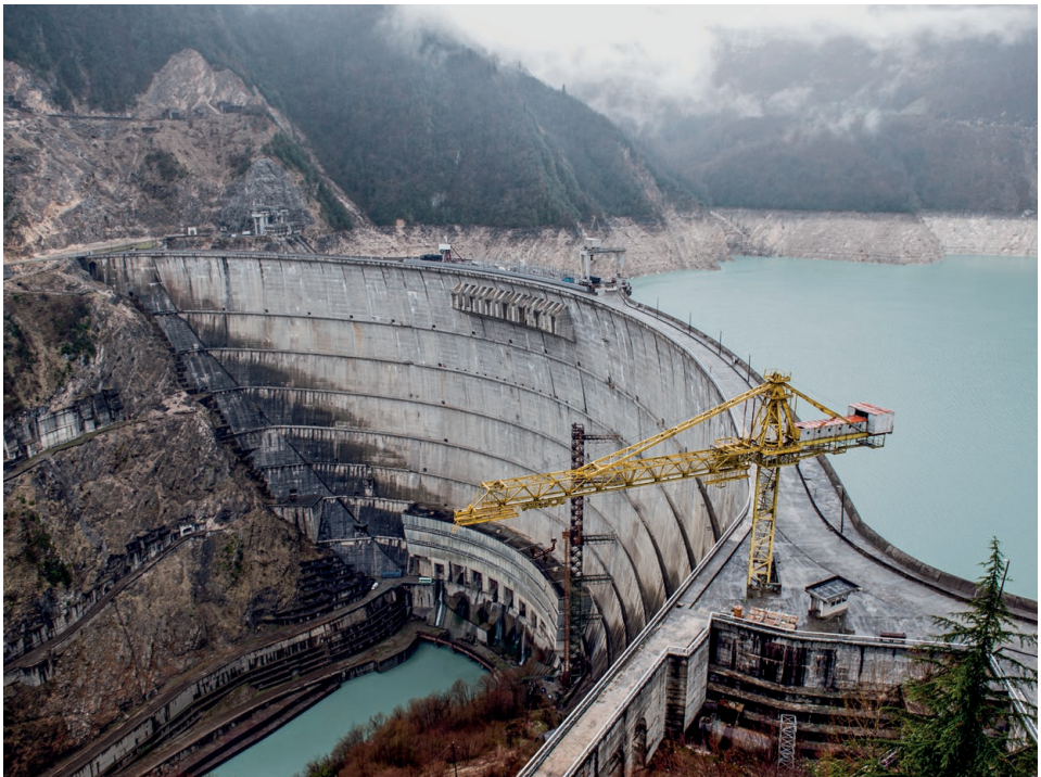
Since 1998 the EBRD has helped to restore and renovate Georgia's Enguri Dam, the world's second largest arch dam. © EBRD
