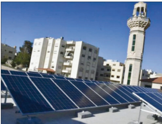
Figure 5: PV system in Al qwasme masjid
